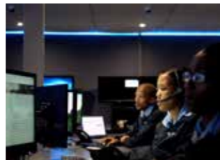
National Control Centre, with off-site Monitoring Capabilities
