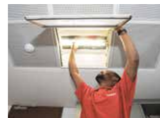
Facilities Management Solutions for Essential Services, e.g. Hospitals and Banks
